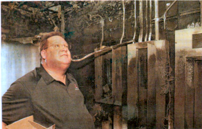
East activities director Ric Powell observes the fire damage in the coach's office at Williams Stadium, located at East 16th and University. MARY CHIND/THE REGISTER
